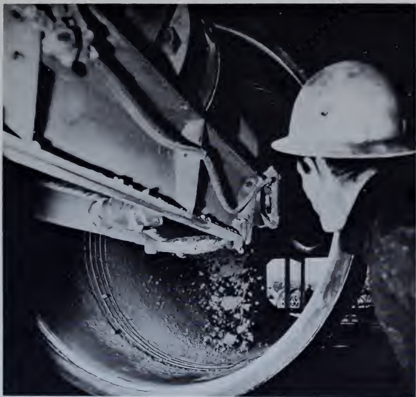
Figure 165.—A centrifugal method of manufacturing concrete pipe in which the concrete is also directly compacted by a steel roller. PX-D-34070.
